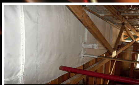
Age Care Centre Vertical Smoke/Flame Barrier
