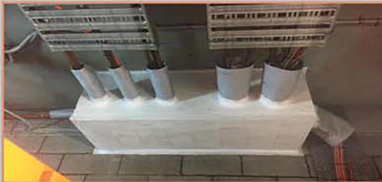
Firefly Intubatt Boxout, installed by an 18 year old female trainee from QLD, under the expert supervision of Archie
